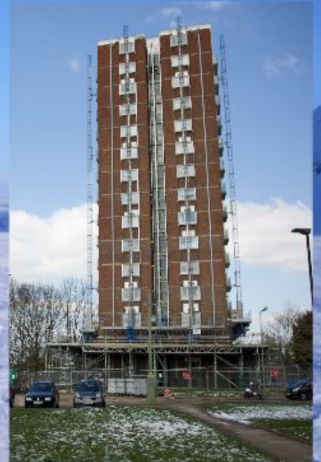
A Granville estate tower block without cladding or insulation last winter
